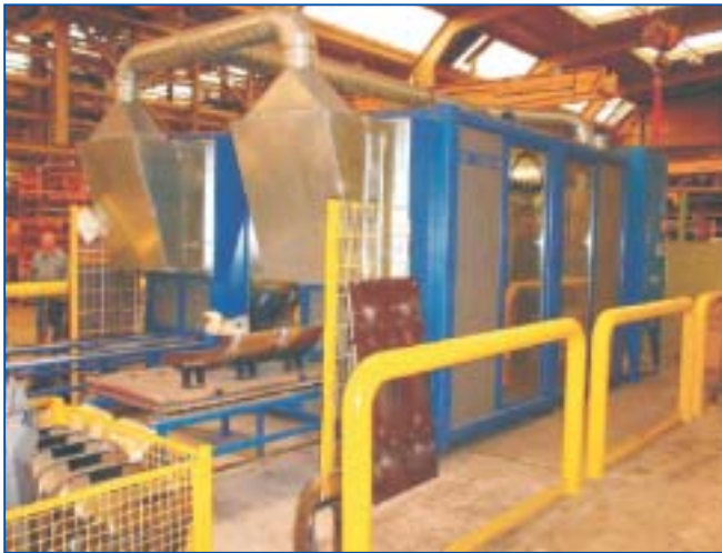
This photo shows a robot cell with ducting from the front and an extractor at the far end.
